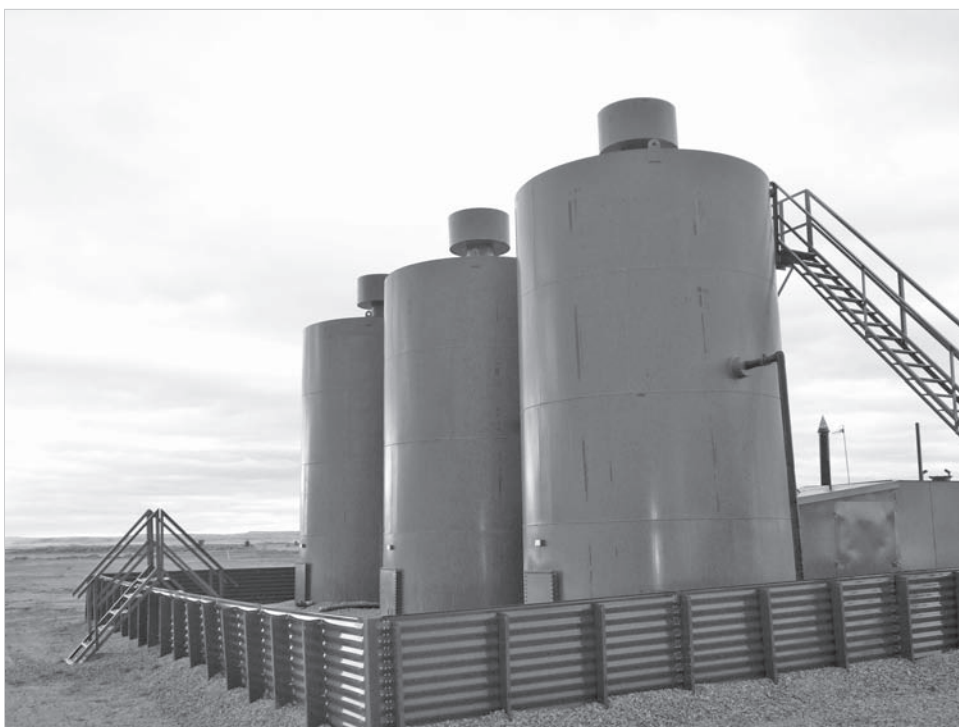
Figure 2: Oil Tanks in Carlsbad, New Mexico
